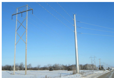
115-kV transmission line | Exponential Engineering
